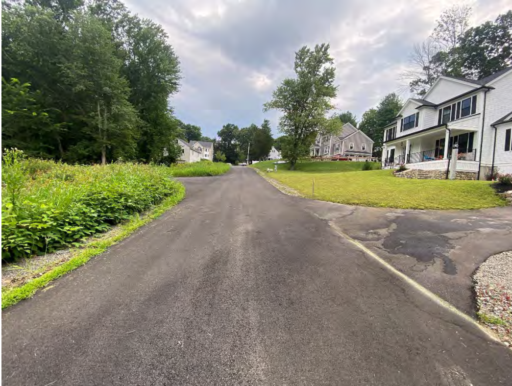
Figure 5 – Status of the extension, from the southern end. Photo taken facing north.
