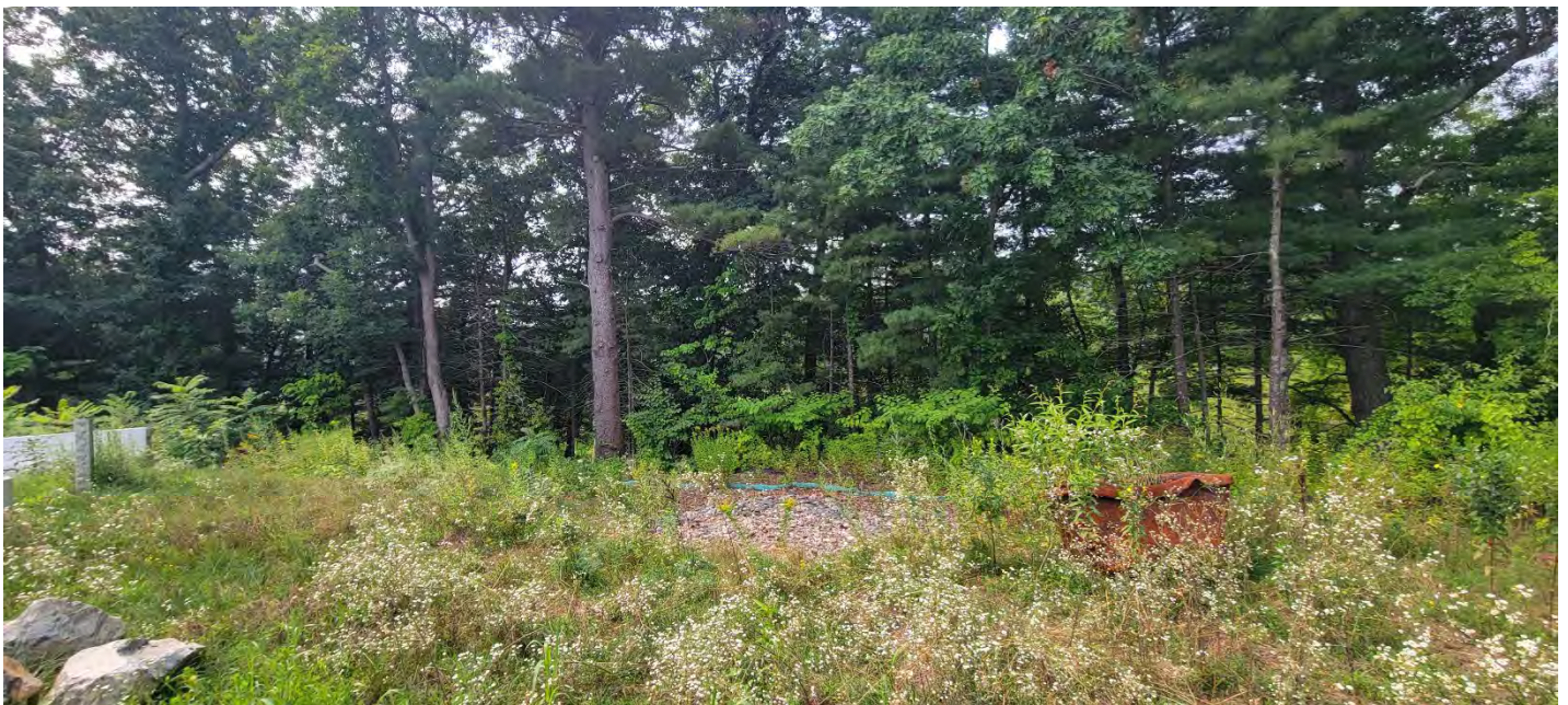
Figure 4 – Sagging silt fence located near the southwestern site limit. Photo taken facing southwest.
