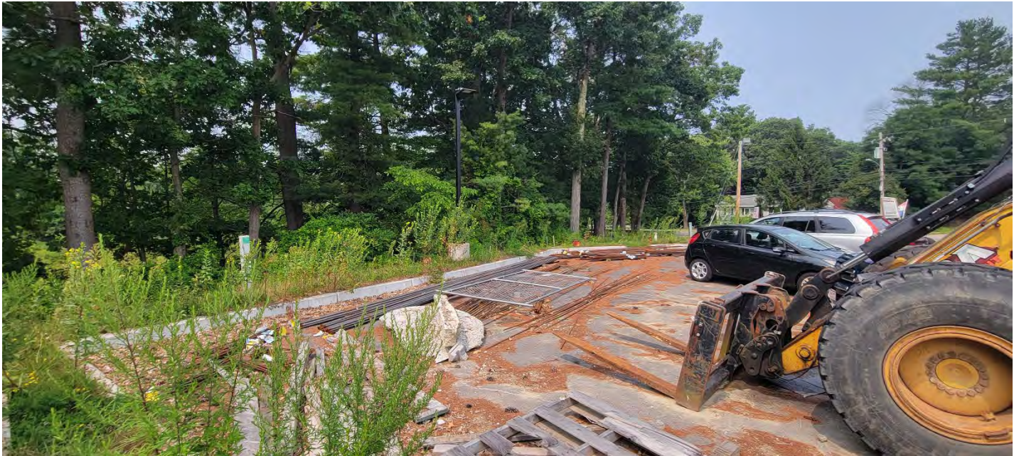
Figure 3 – Status of the stockpiles near the southwest corner of the site. Photo taken facing north.
