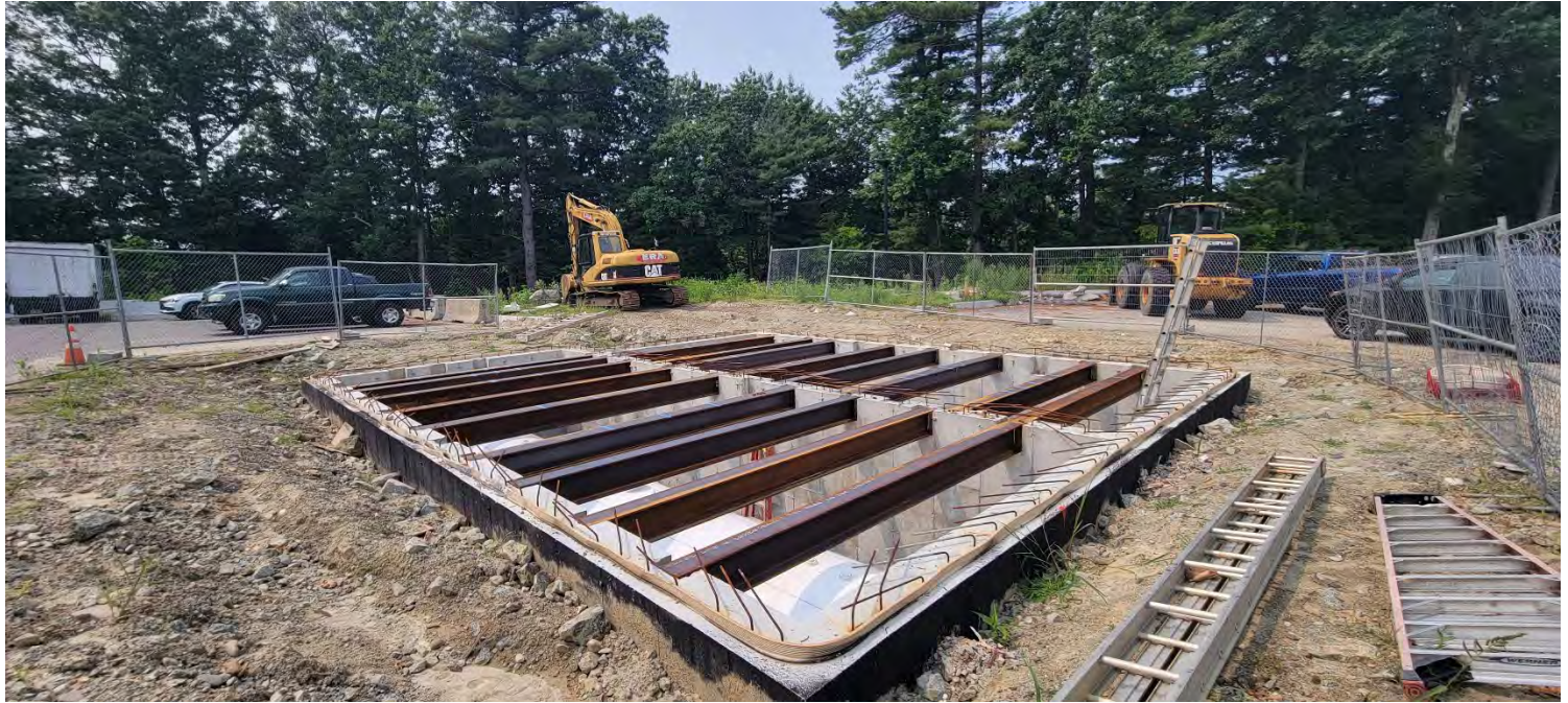
Figure 1 – Status of eastern vault section, installed I-beams, and construction fencing. Photo taken facing southwest.
