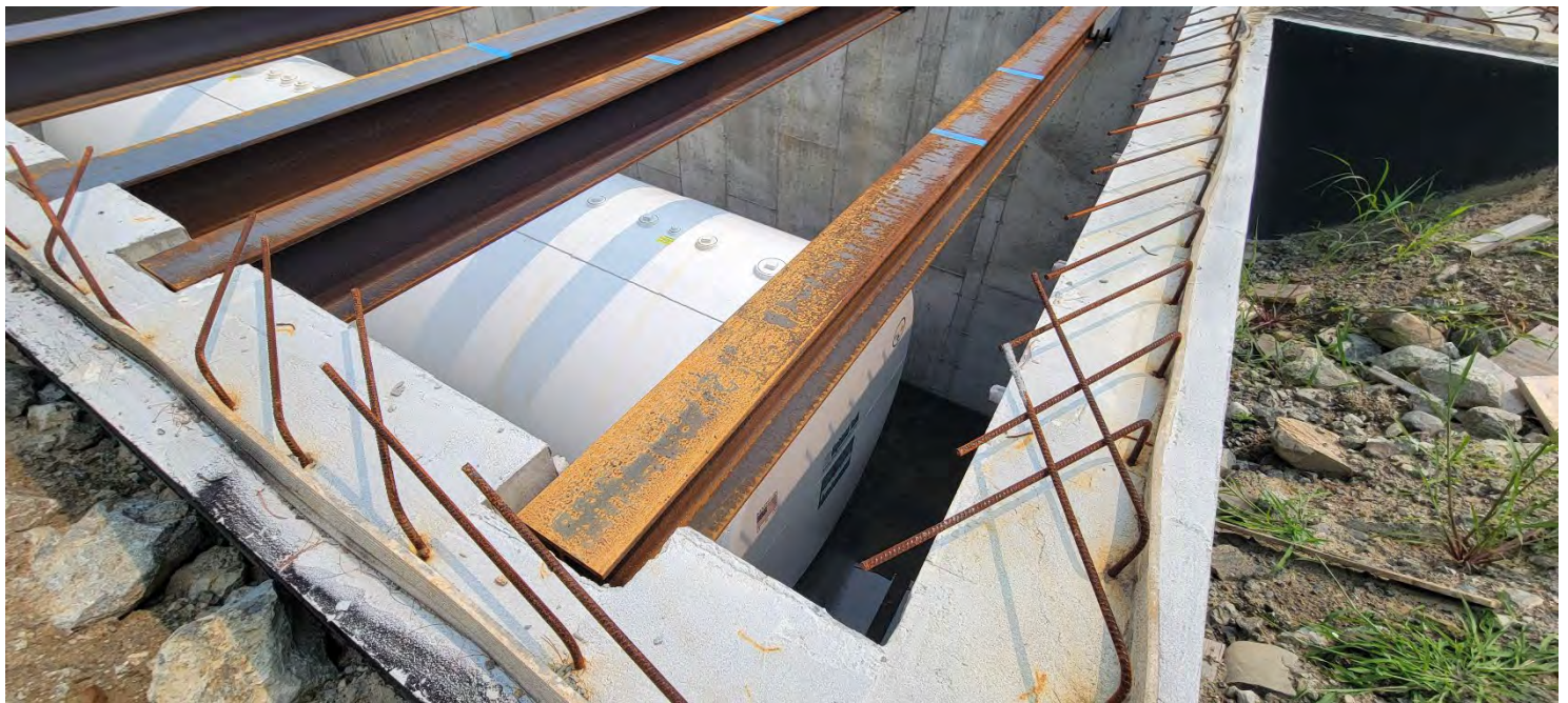
Figure 2 – Status of western vault section. Water build-up was observed within the vault. Photo taken facing northeast.
