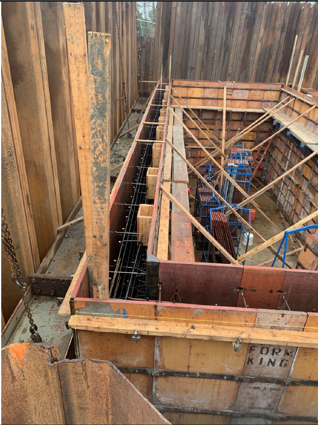
Figure 4 – Rebar within formwork of the eastern wall of the 12,000-gallon tank bay. Photo taken looking south.
