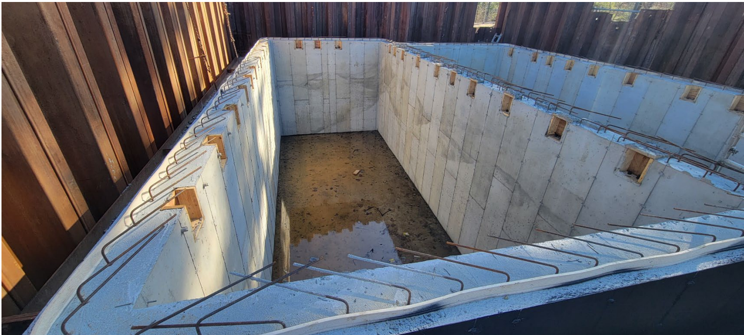
Figure 2 – Status of eastern vault section at the “end” of the water-tightness test. Photo taken facing south.
