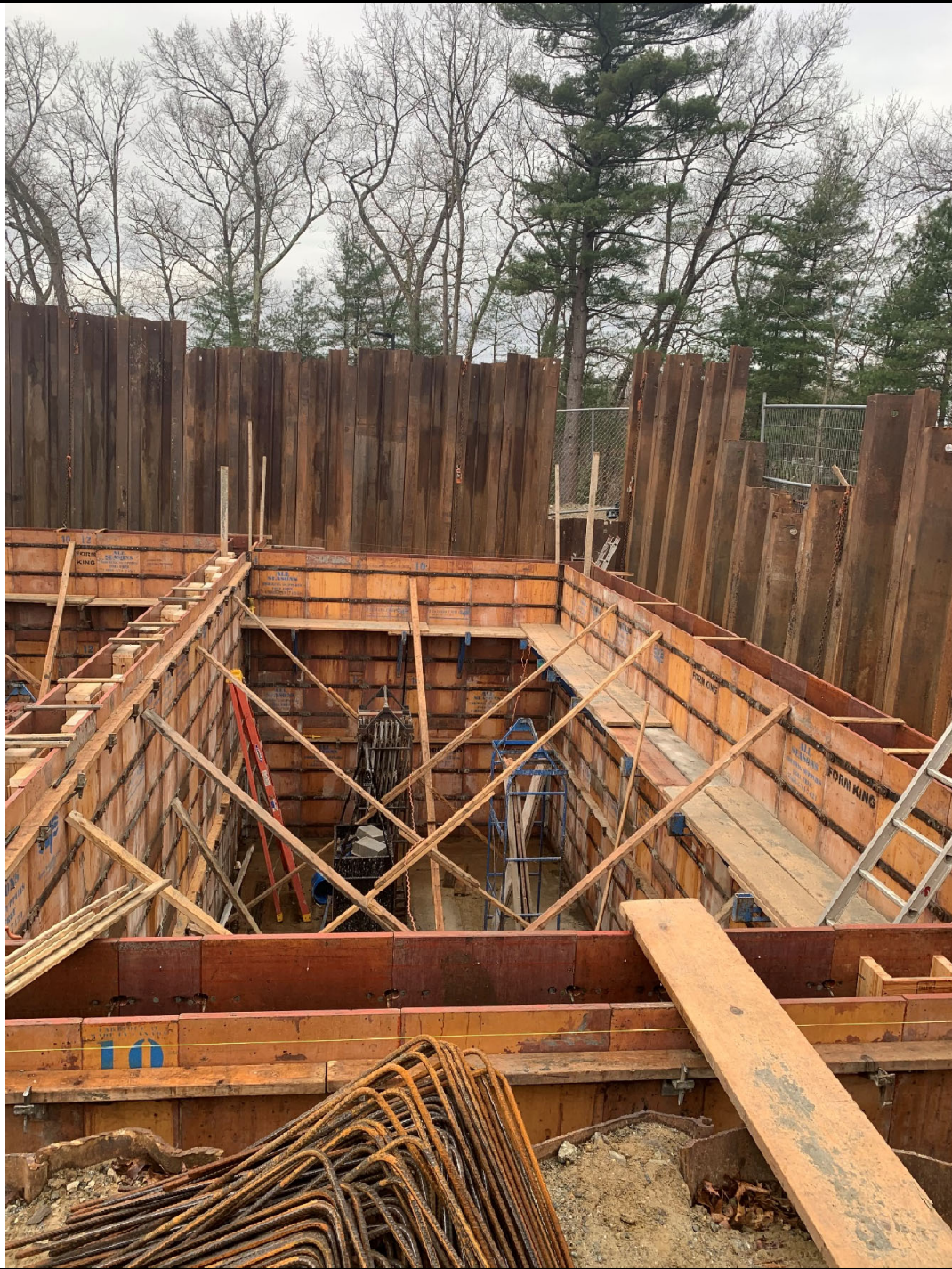
Figure 3 – 10,000-gallon tank bay, formwork in place for concrete pour. Photo taken facing south.
