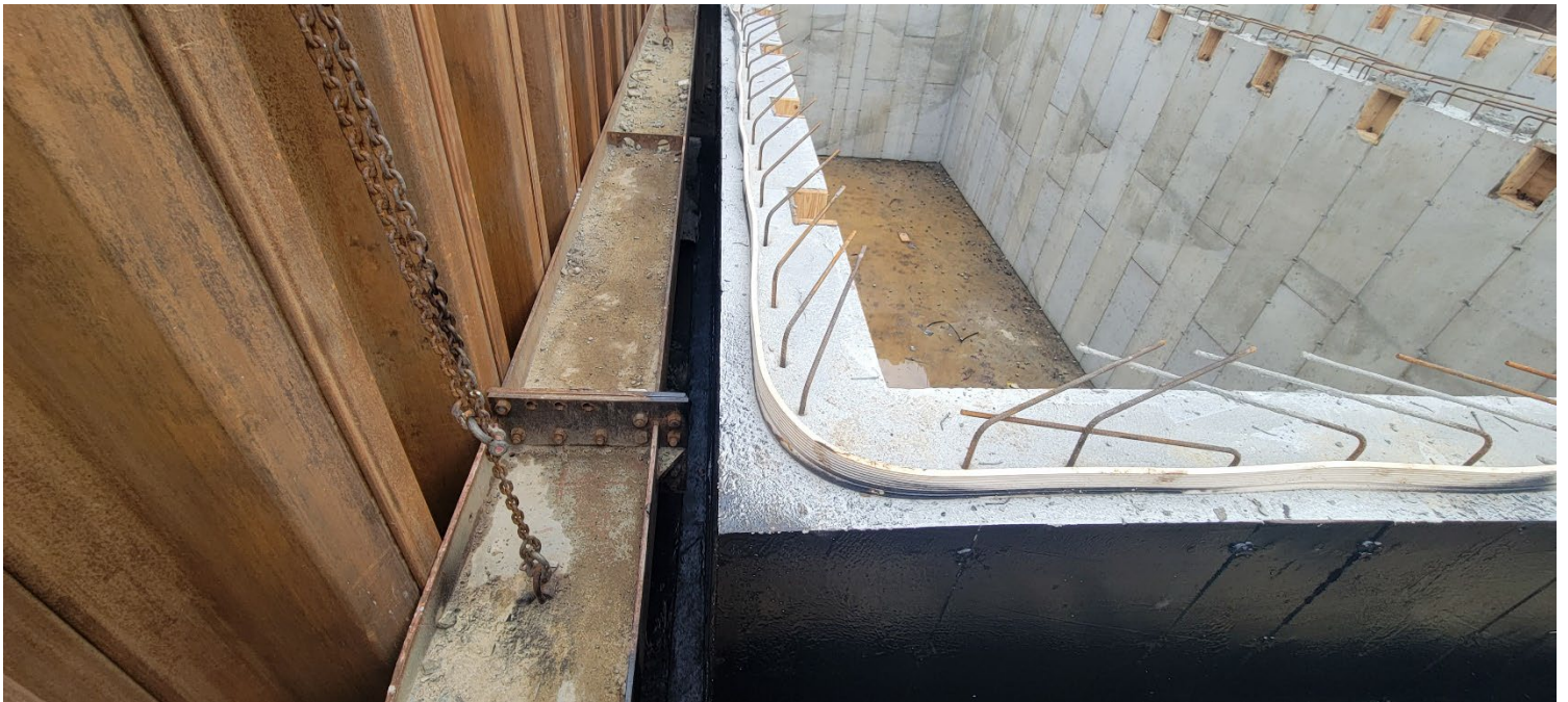
Figure 2 – Existing water build-up east of the foundation footing (<2") and existing water build-up within the eastern section of the vault (<1"). Photo taken facing south.
