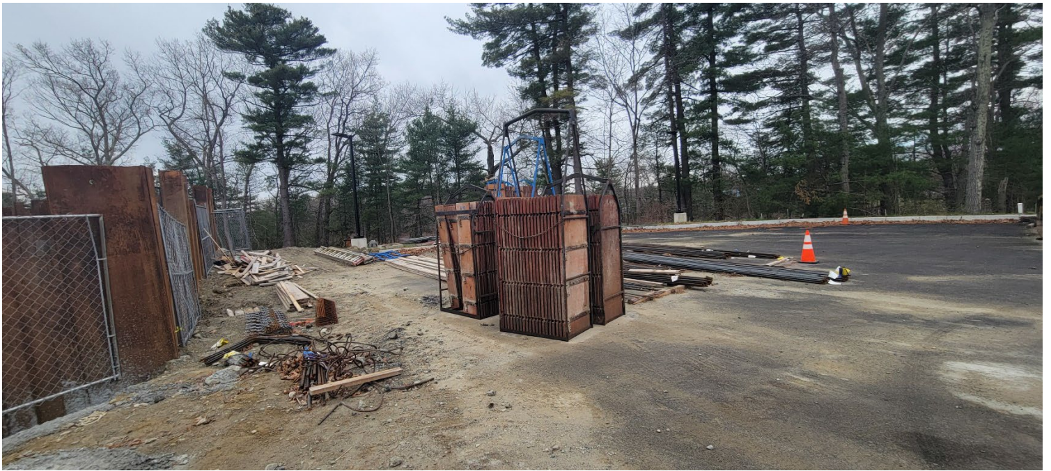
Figure 4 – Rebar and concrete form stockpiles west of the existing vault. Photo taken looking southwest.
