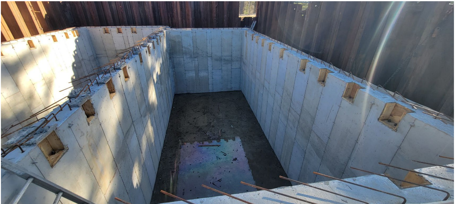
Figure 4 – Status of western vault section at the “end” of the water-tightness test. Photo taken facing south.
