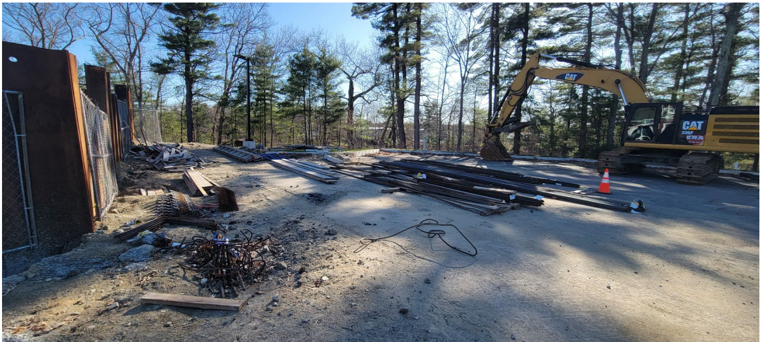
Figure 6 – Status of rebar and concrete form stockpiles northwest of the vault. Photo taken facing southeast.
