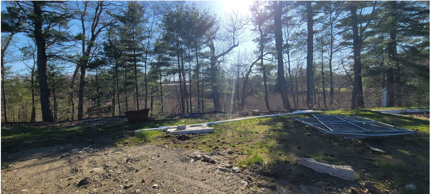
Figure 7 – Sagging silt fence located near the southwestern site limit. Photo taken facing southwest.
