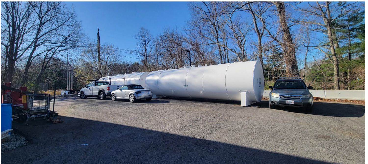
Figure 8 – Stockpiled proposed gas tanks to be placed in vault, south of existing garage. Photo taken facing southeast.
