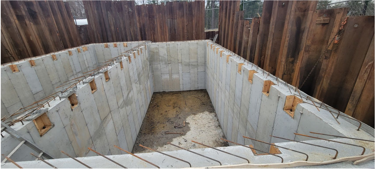
Figure 3 – Status of the western portion of the concrete vault. Photo taken facing south.
