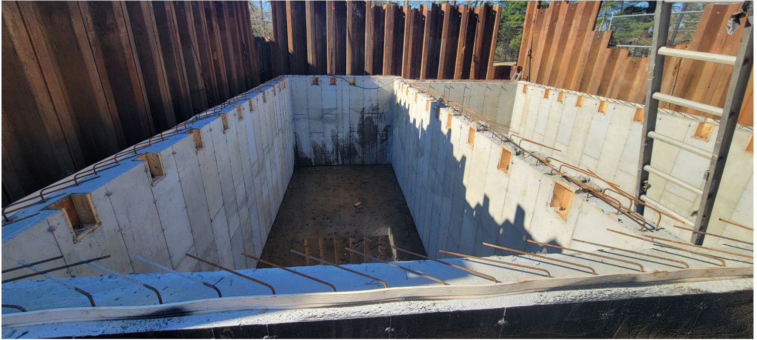
Figure 1 – Status of eastern vault section following water being added to start the water-tightness test. Photo taken facing south.
