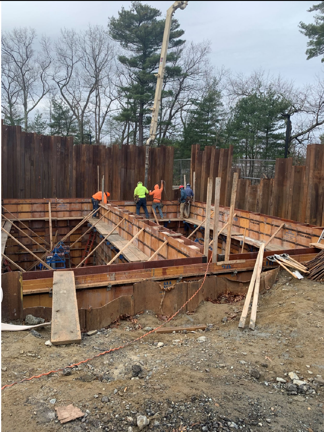
Figure 1 – Overview of concrete pour area. Formwork set to pour concrete vault walls. Concrete being poured into the southern wall of the 10,000-gallon bay shown. Photo taken facing southwest.
