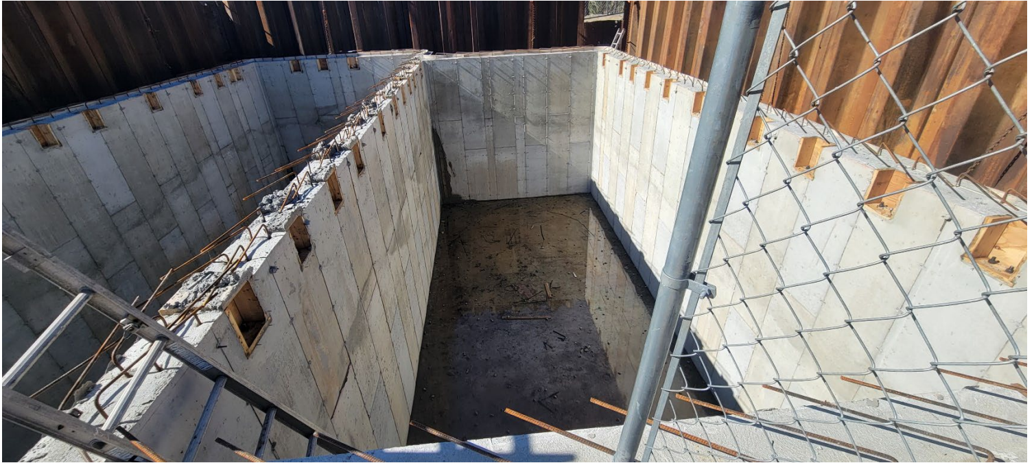
Figure 3 – Status of western vault section following water being added to start the water-tightness test. Photo taken facing south.
