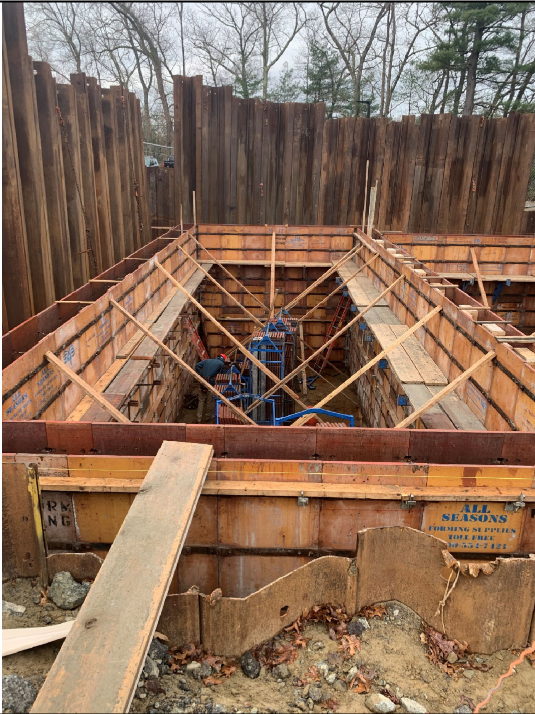
Figure 2 – 12,000-gallon tank bay, formwork in place for concrete pour. Photo taken facing south.
