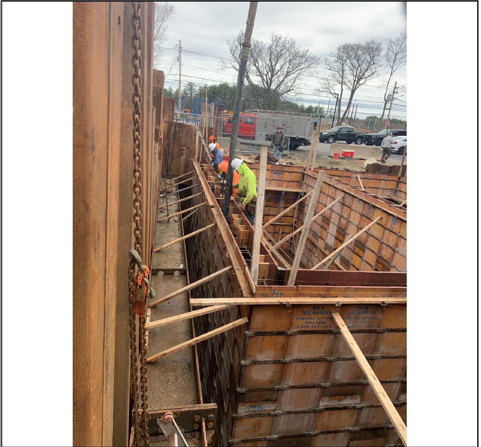
Figure 5 – Western wall of 10,000-gallon tank bay shown being poured and vibrated. Photo taken looking northeast.
