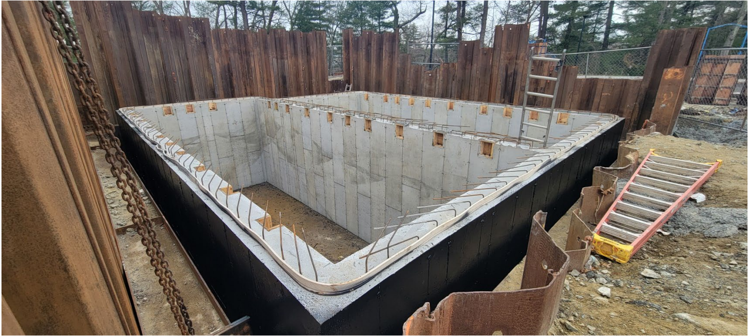
Figure 1 – Overview of the open excavation, previously poured wall sections, waterproofing along the outside limits of the foundation, and rebar at the top of the structure. Photo taken facing southwest.
