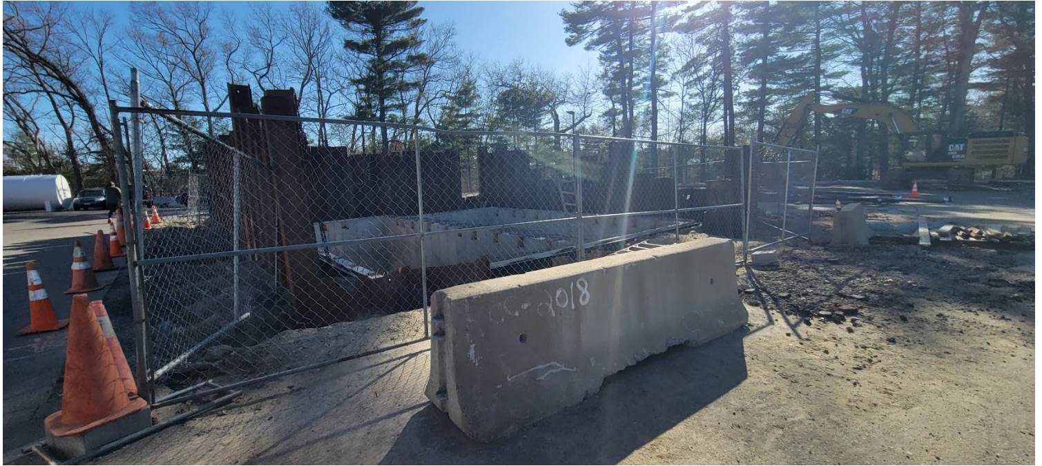
Figure 5 – Overview of the concrete vault, fencing, metal shoring, and nearby equipment on site. Photo taken facing southwest.
