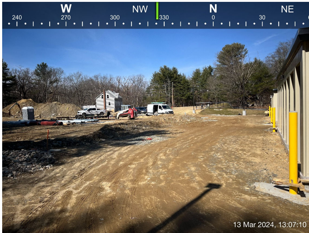
Photo #11: Looking towards Salem Street from southwest corner of Building #3. Stabilized, compacted gravel surface in place in areas under Phase 1.
