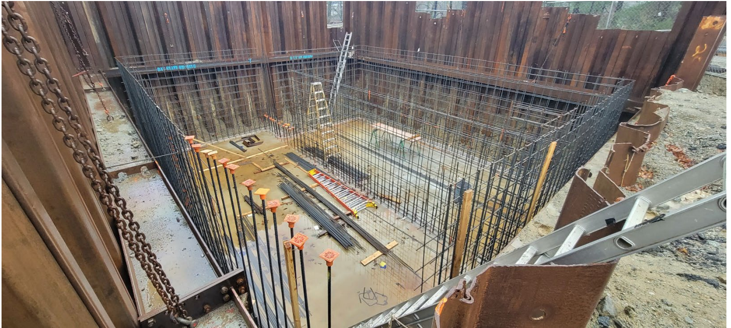
Figure 1 – Overview of the open excavation, previously poured floor, and assembled wall rebar sections for the proposed concrete vault. Photo taken facing southwest.
