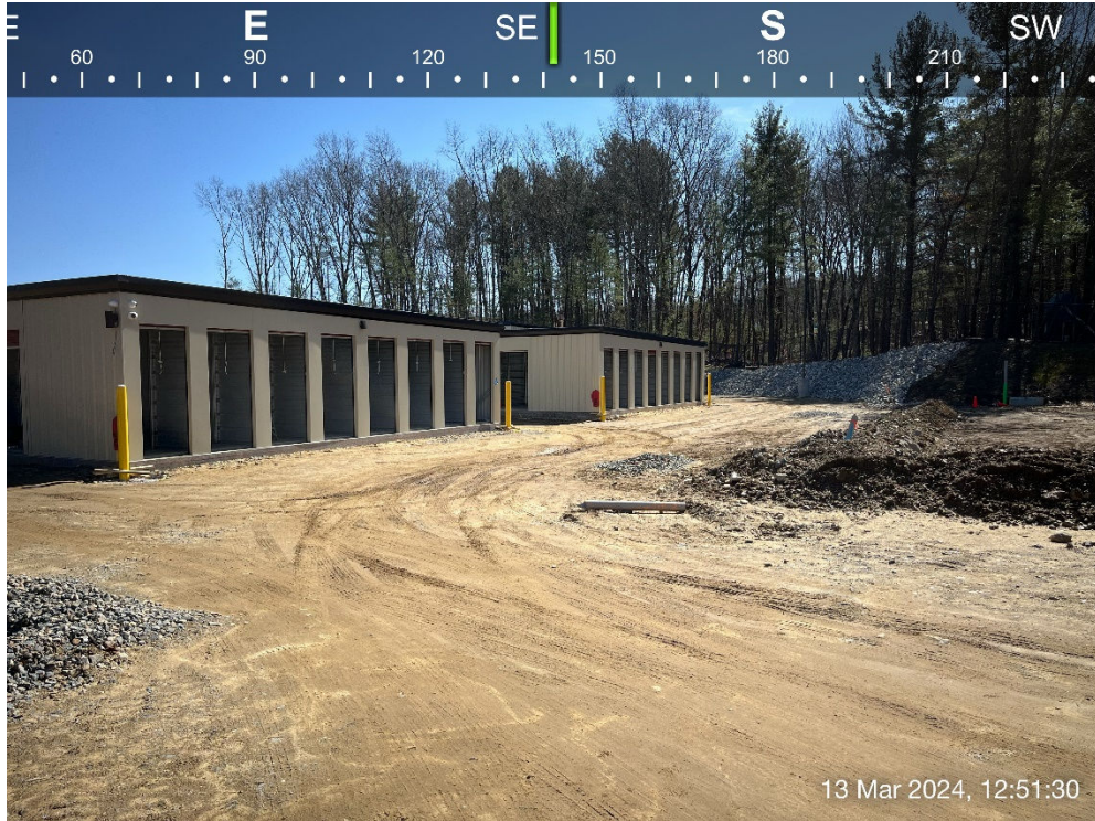
Photo #12: Looking towards west end of Buildings #3 & #4. Stabilized, compacted gravel surface in place in areas under Phase 1.
