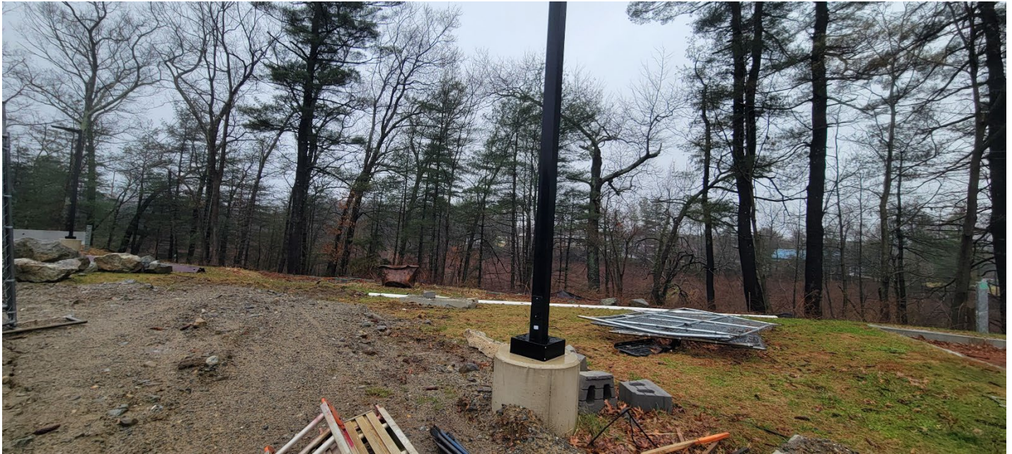
Figure 5 – Sagging silt fence like located near the southwestern site limit. Photo taken facing southwest.
