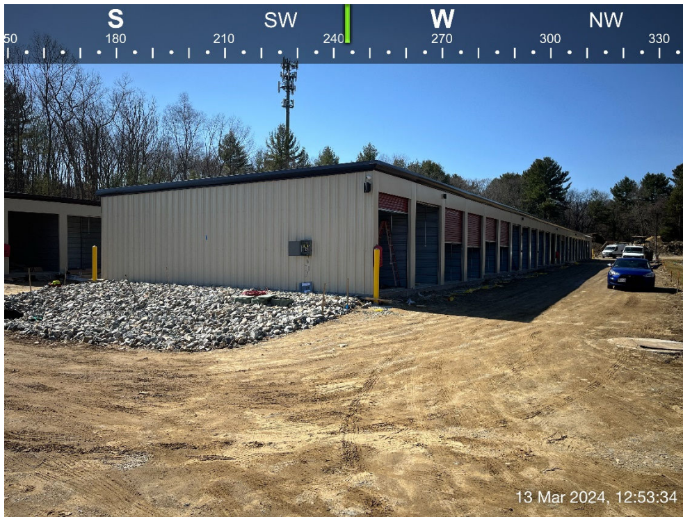
Photo #5: Looking along north side of Building #2. Stabilized, compacted gravel in place.
