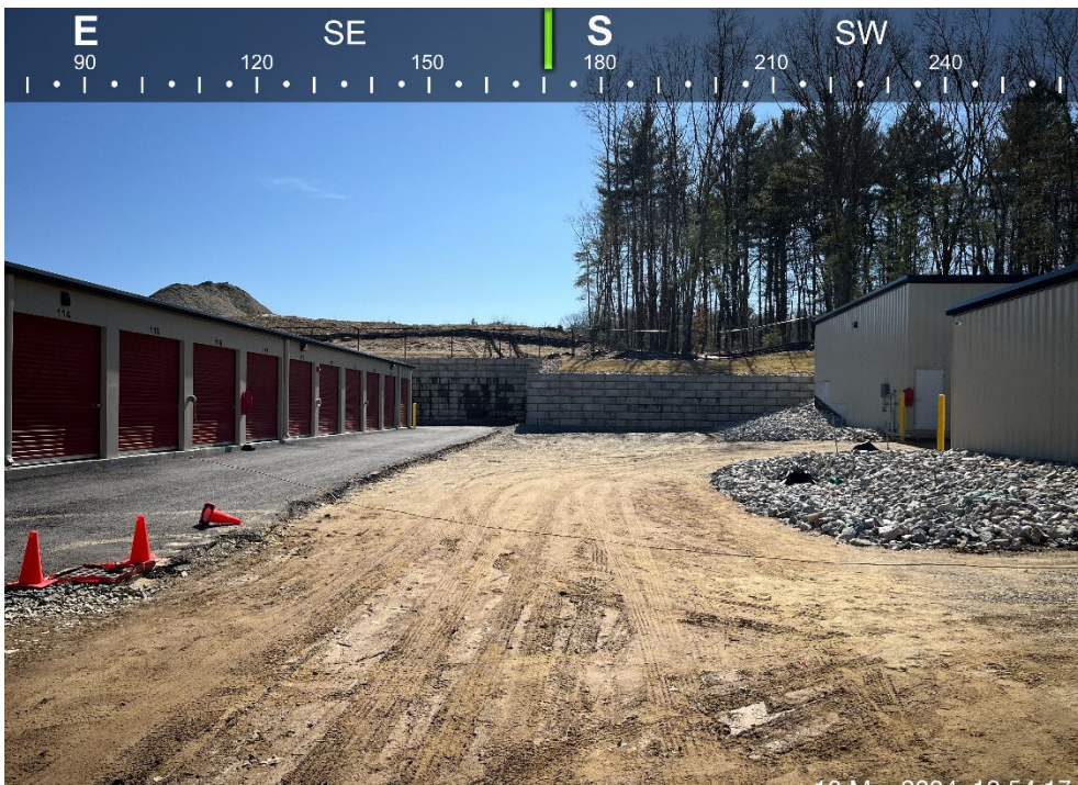
Photo #6: Looking at area between existing storage facility and tie-in points. Grassed medians on east side of Buildings 2, 3 & 4 have been replaced with large diameter rip rap to cut down on maintenance and stabilization/slope concerns.
