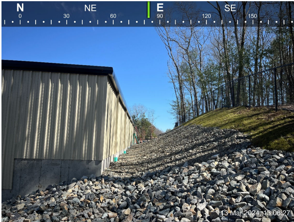
Photo #10: Looking behind Building #4. Stone stabilized slope in combination with upper grassed slope.
