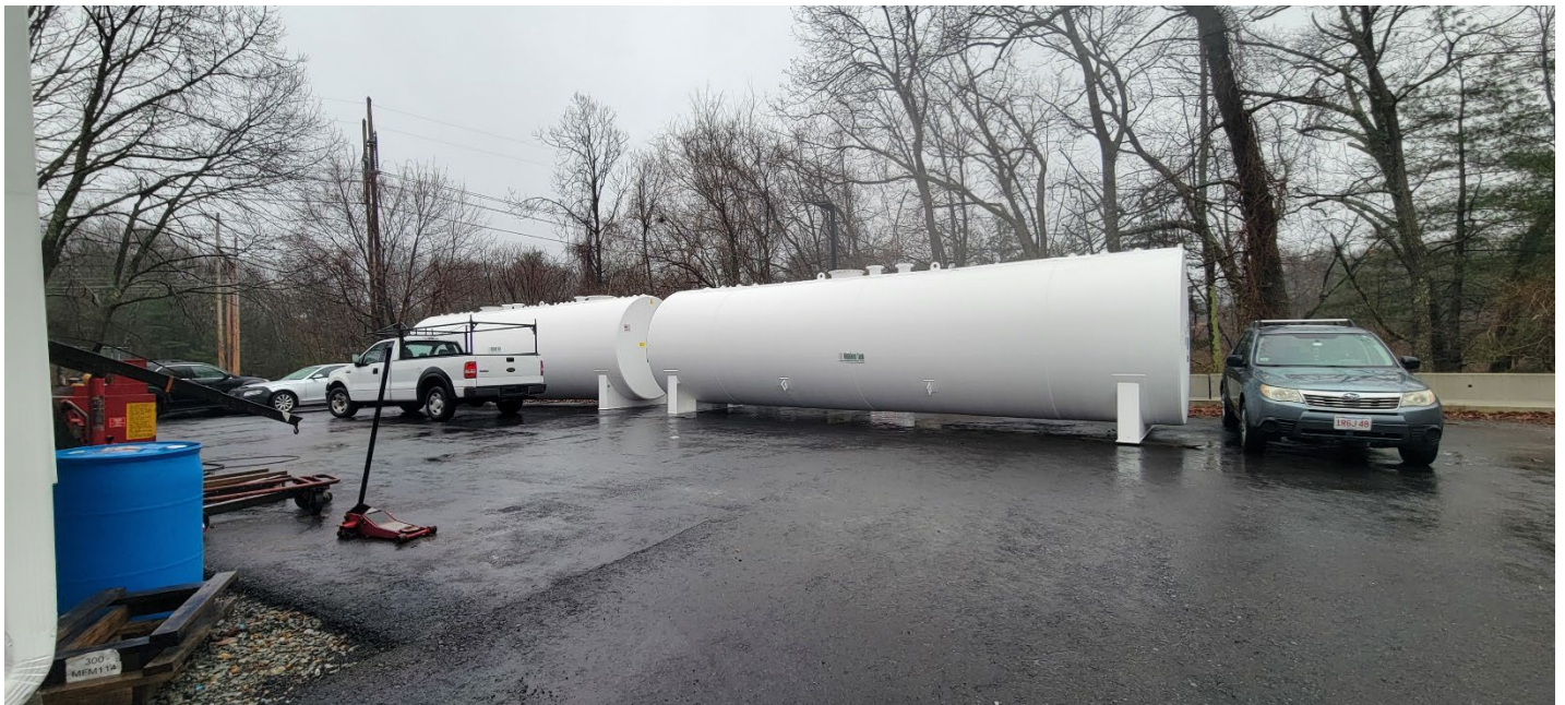
Figure 6 – Stockpiled proposed gas tanks to be placed in vault, south of existing garage. Photo taken facing southeast.
