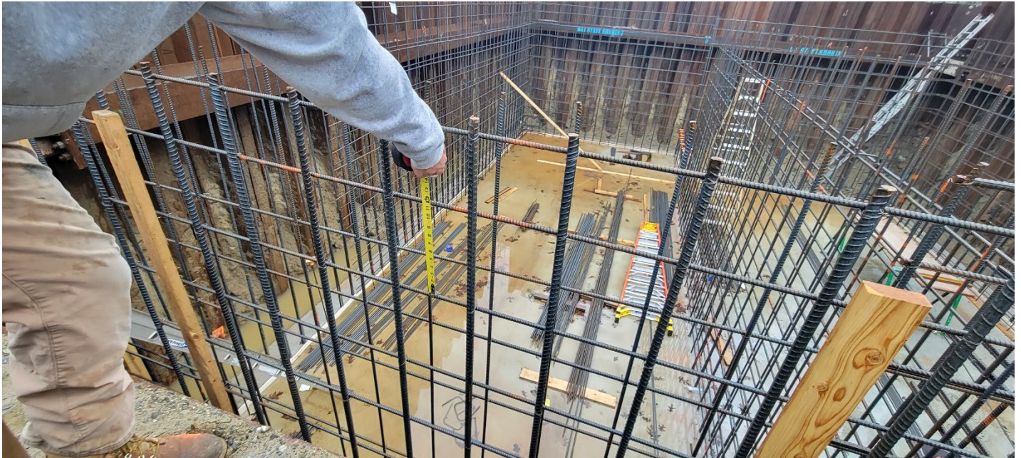
Figure 3 – Example measurement of the “exterior” horizontal bar (#4) spacing. Photo taken facing south.
