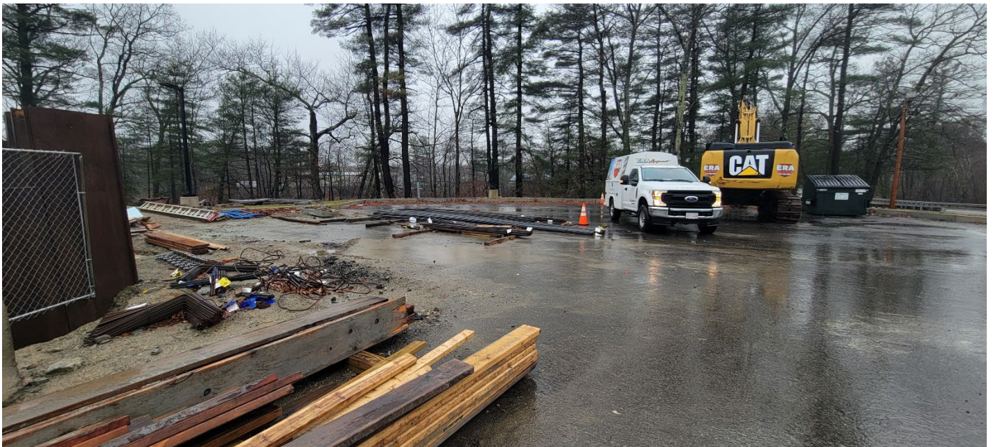
Figure 4 – Rebar and other construction material stockpiles located near the open excavation. Photo taken facing southwest.
