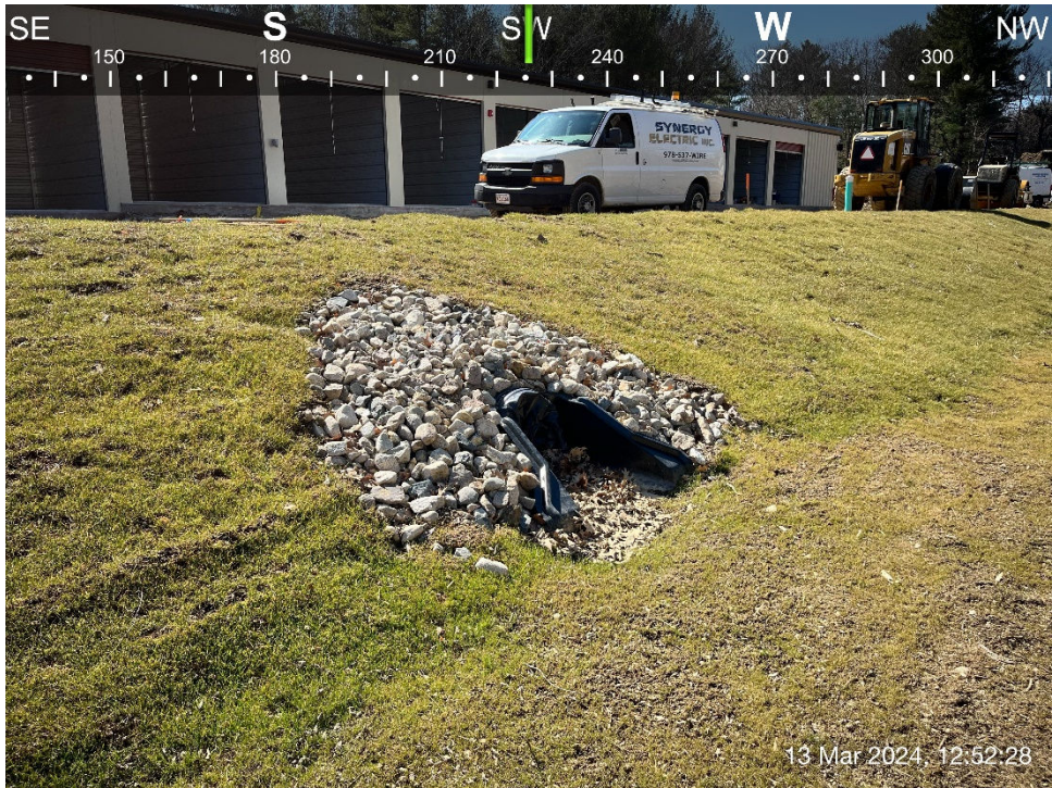
Photo #3: Inlet/outlet FES to Chamber System #1 (one of two inlet/outlets)
